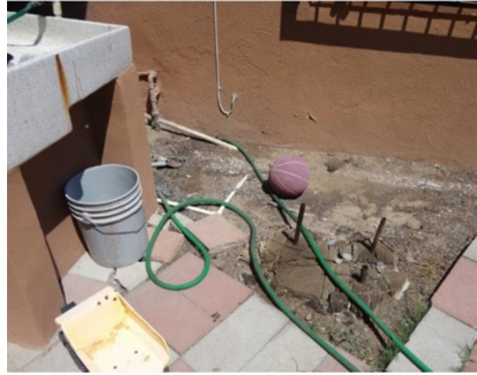
Steel pipes poking out of the ground in an outside play area. Source: Department of Health and Human Services, Office of the Inspector General
