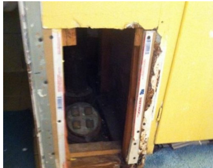
Hole in bathroom wall exposing pipes. Source: Department of Health and Human Services, Office of the Inspector General
