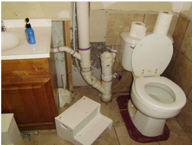
An unfinished bathroom with exposed pipes that was used by children.
