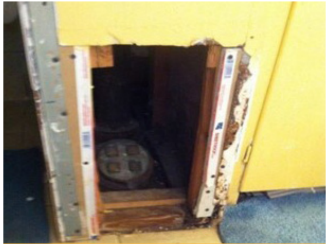
Hole in bathroom wall exposing pipes.
