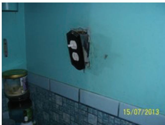
An electrical outlet protruding from the wall and covered with duct tape.
