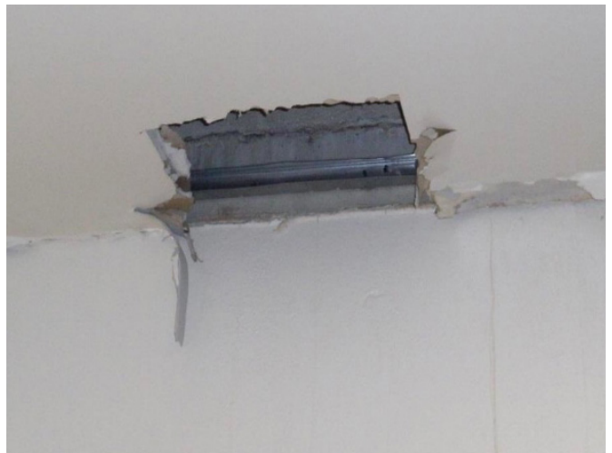
A hole in the ceiling and paint peeling in the all-purpose room showed that the area was in poor repair.
