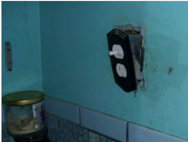
An electrical outlet protruding from the wall and covered with duct tape. Source: U.S. Department Health and Human Services Office of the Inspector General.
