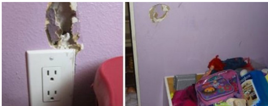
Holes in the wall within a child’s reach. Source: U.S. Department Health and Human Services Office of the Inspector General.
