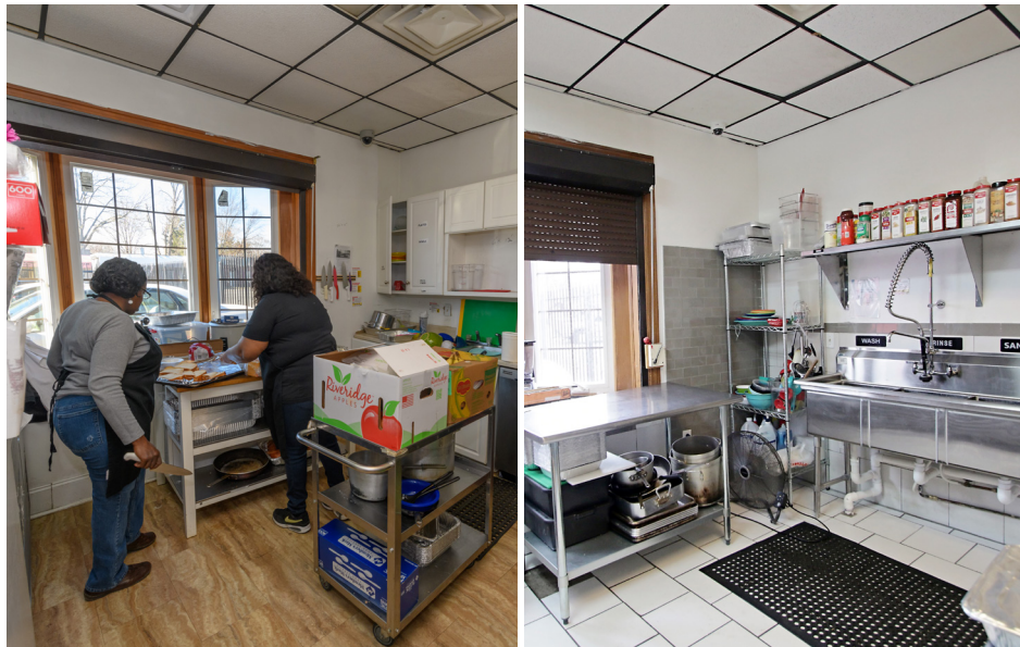
Renovation of the Little Scholars Child Development Center (before and after). Photo provided by IFF.
