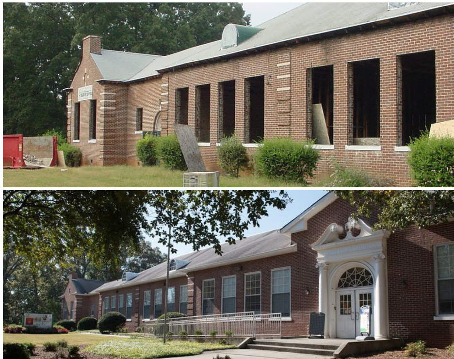
Renovation of a closed school building into an early learning center. (before and after) Photo provided by Early Learning Property Management.
