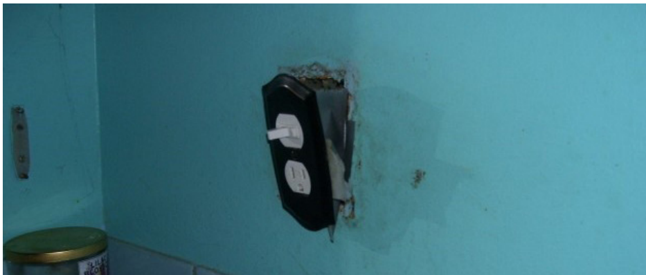
An electrical outlet protruding from the wall and covered with duct tape. Source: U.S. Department of Health and Human Services' Office of the Inspector General.
